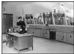
Gotland 1 Control Room 20 MW mercury valves
