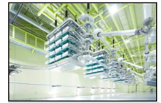
Xiangjiaba - Shanghai 800 kV Classic 6 400 MW
